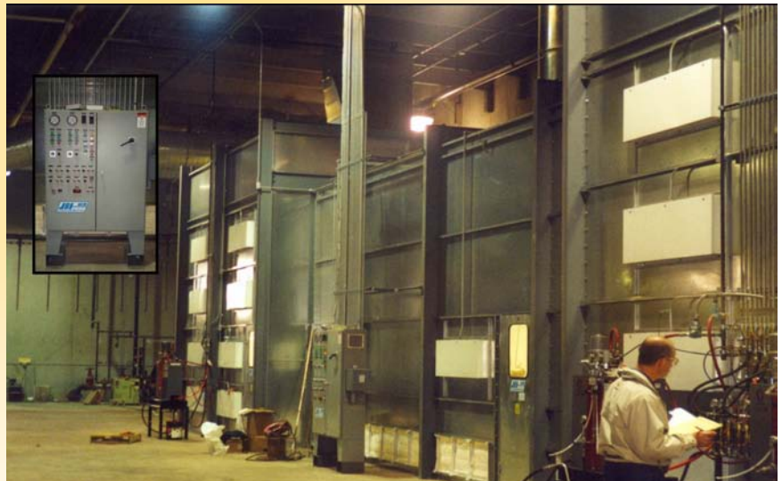
Downdraft booths and flash tunnel
